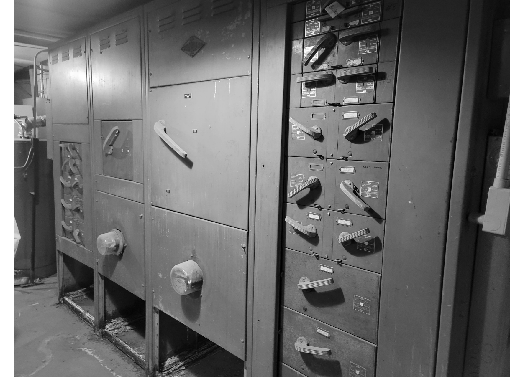
2 EXISTING ELECTRICAL GEAR ES101 NOT TO SCALE
